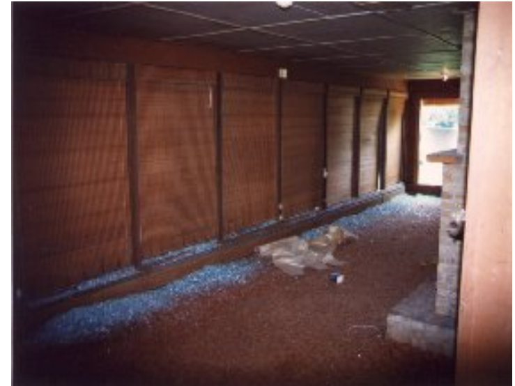
Sunroom Before - note the long pile of broken glass by the outside wall.
