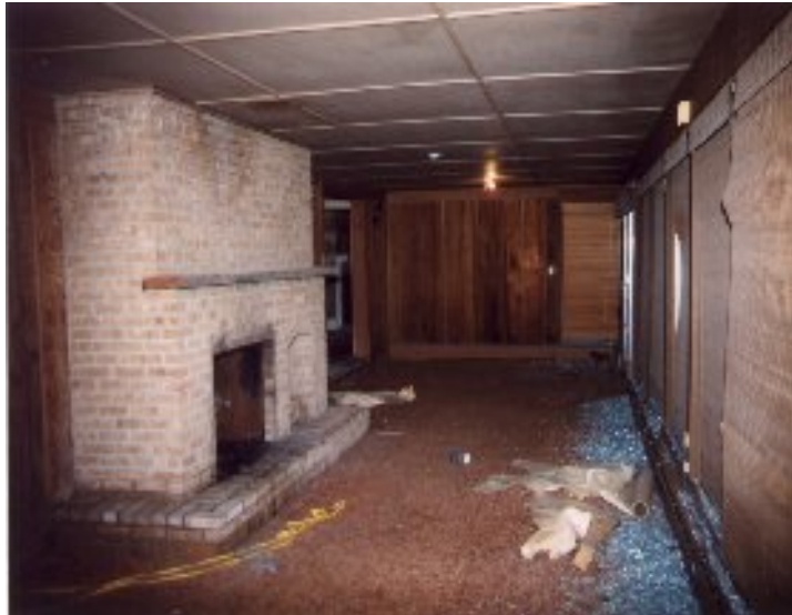
Sunroom - All the patio doors and large windows were broken out except for one.
